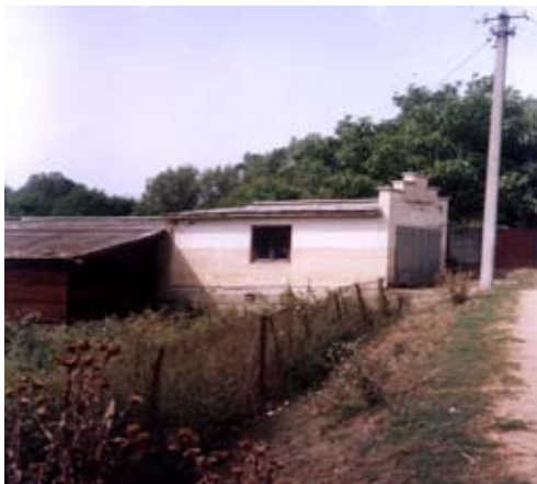
Fig. 3. Level of flood on the wall of the building in March 2001
